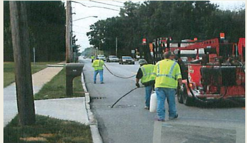
Crack and Joint Seal
